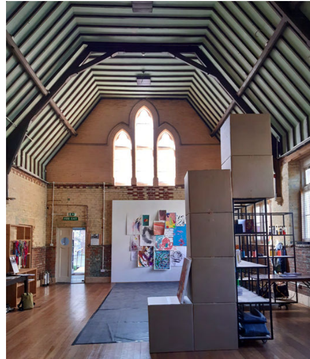
1. Main Hall looking West: arched windows to gable end and vaulted soffit with timber purlins
