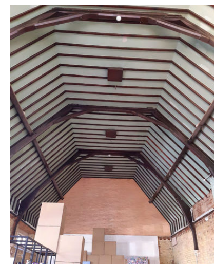
8. Structural issues of existing roof and poor thermal envelope
